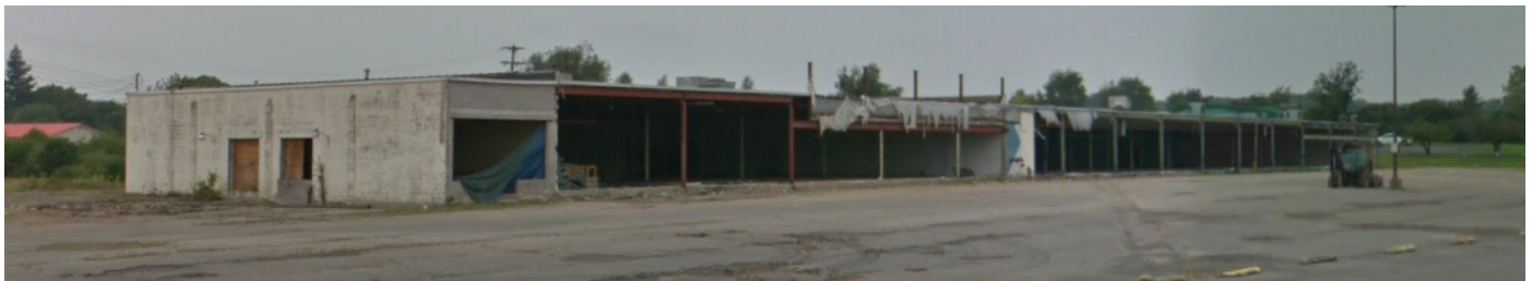
Condition of the existing building is critical to the viability of the site. Further investigation is needed.
